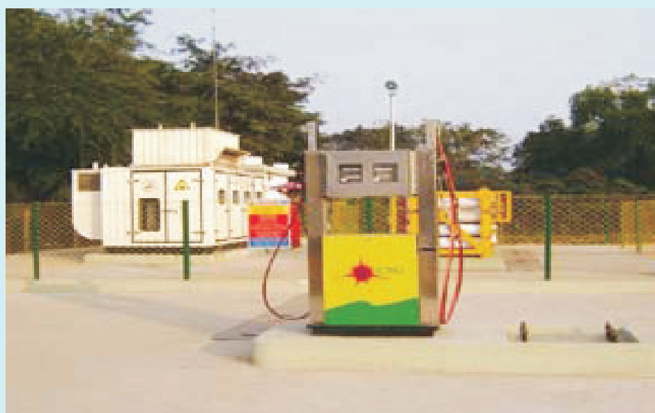
CNG METERING STATION AT GGS SITE
